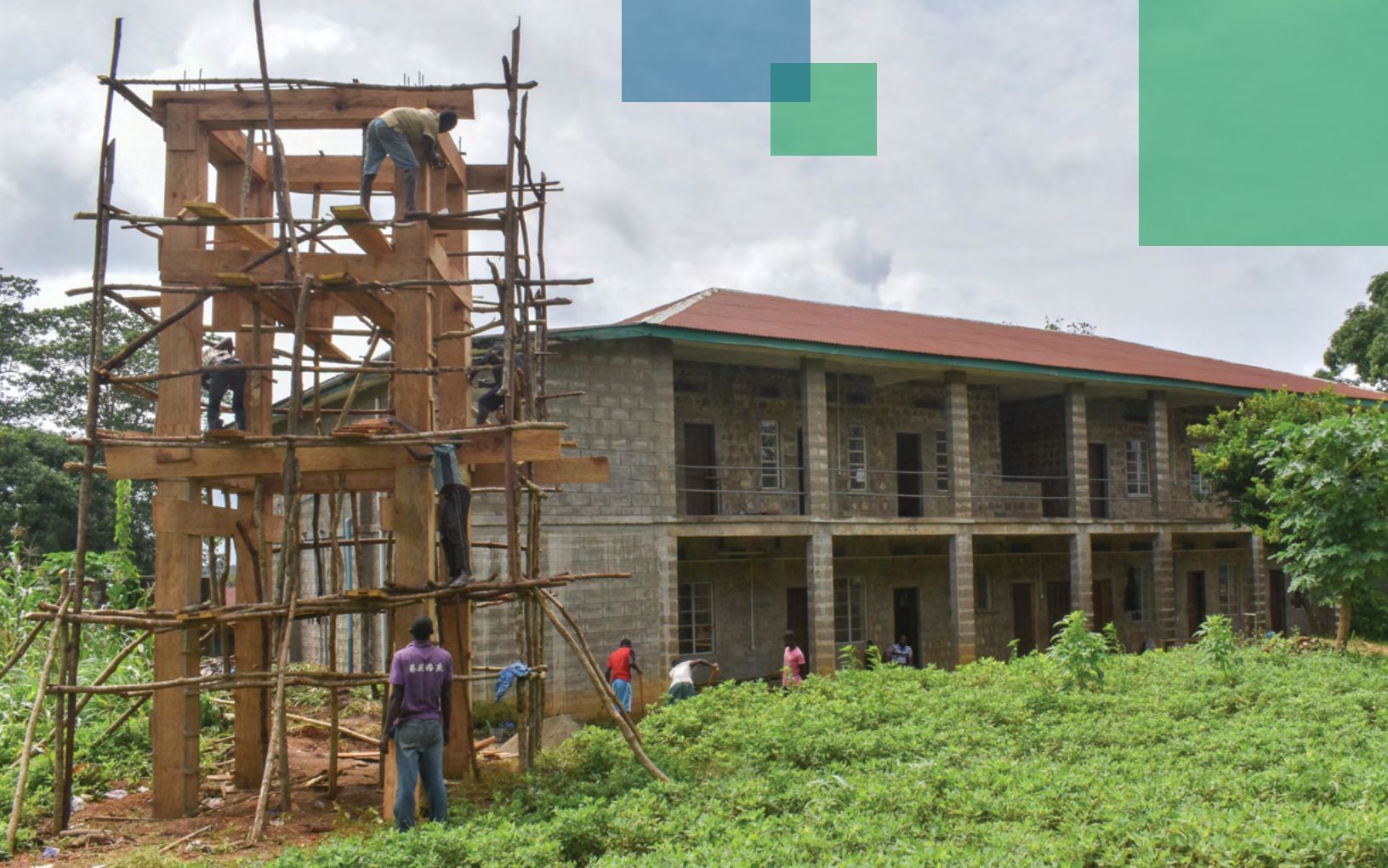
Above Image: Workers construct a platform for a water tank at the converted quarantine center at Nixon Memorial Hospital
